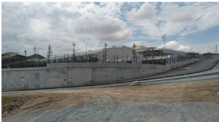
New Fruit-Vegetable Marketplace under construction and School on the South of the site
